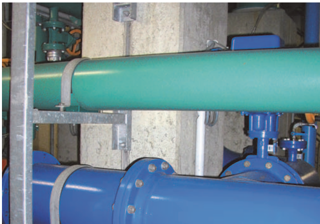
Pipe supports on vertical HZA Channels
